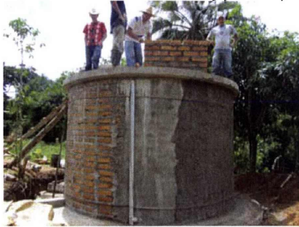
Water Tank built by team led by SHPE in Binghamton in Rio Hondo, Honduras
